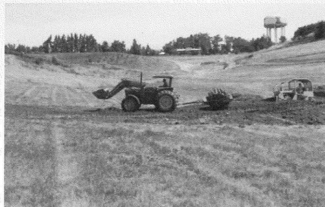
Excavating the upper pond and compacting its dam. July, 1986. Note the sparse vegetation, compared with the lush plantings that are now established in the arboretum in 2007.
