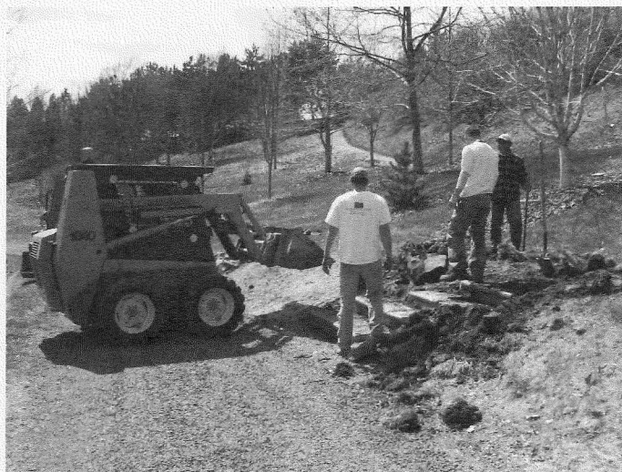
Workers install historic steps in the Robert Seale Mugo pines collection. Paul Warnick photo
