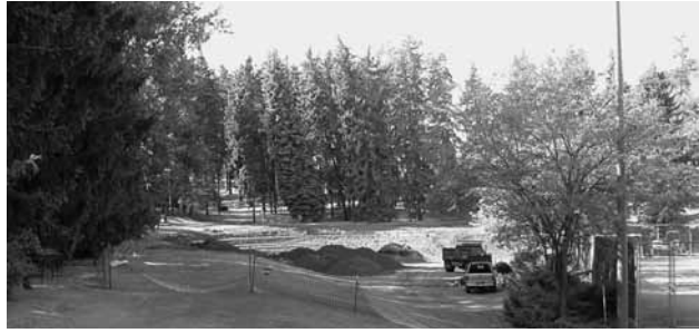
Looking west toward the Shattuck Amphitheater, summer 2002, amphitheater renovation is under way. Charles Zillinger photo.
