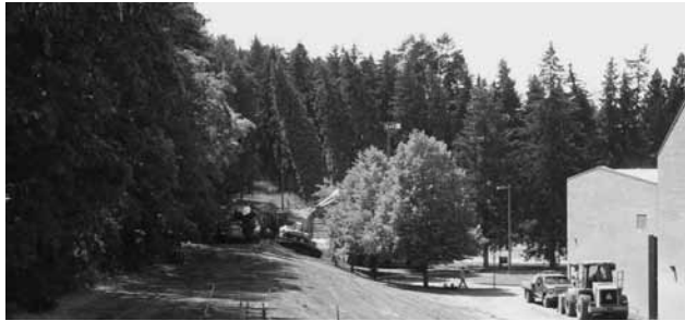
Looking west toward the Shattuck Amphitheater, summer 2009, new chilled water line installation is underway. Charles Zillinger photo.
