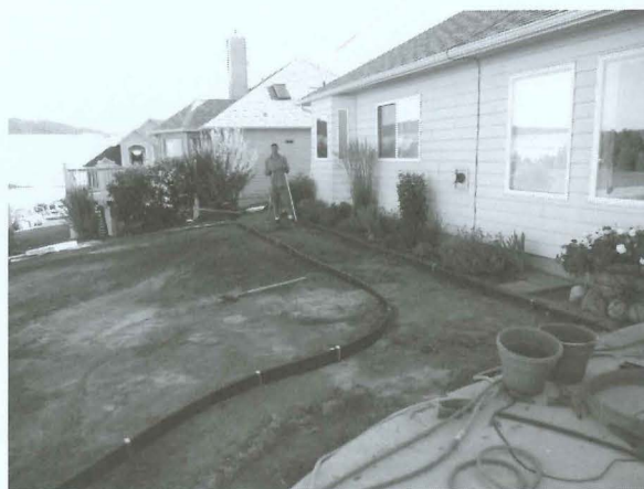
Don Regan works on installing framing for upper path. Photo by Maureen Regan
