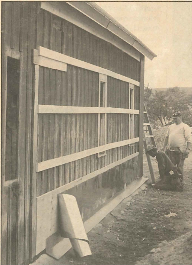
Mike Amos (back) and Jeff Bosse (front) install protective steel siding to the north side of the Arboretum barn, September 26, 2001.
