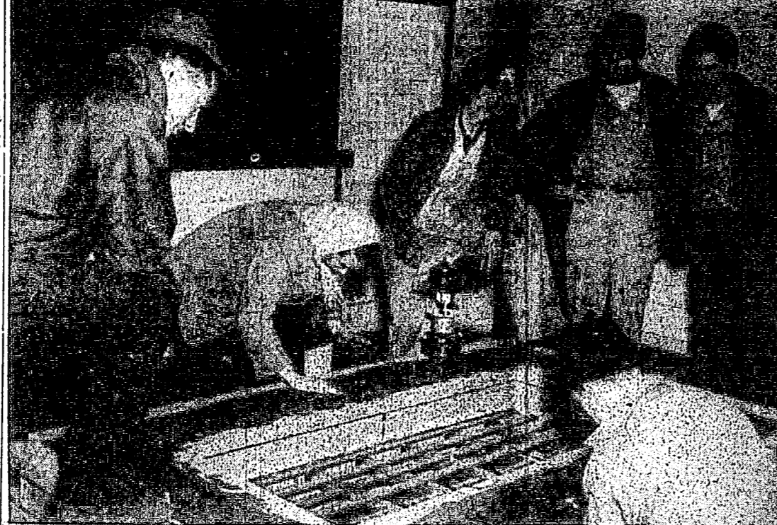
Bonnie Kuehl, secretary of the Vandal Ski club, places small rocks in wet cement to spell out the numerals "1946" while other members of the club gather to watch completion of part of the work on the lodge. Weekly work parties have been numerous enough so that a housewarming can probably be held in January, Jack Numbers, president, has revealed.
