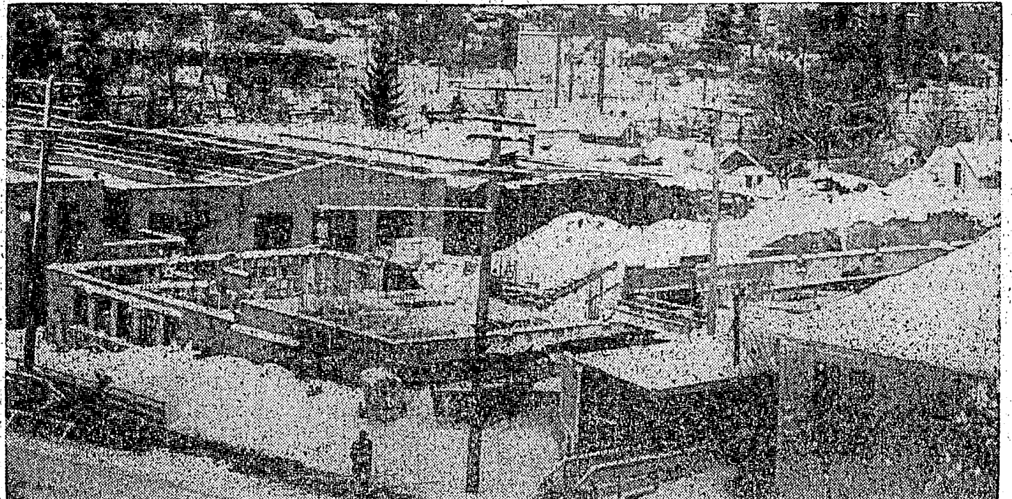
Old man winter has done but little in the blowing down of the building program which was inaugurated last spring. In the foreground workers dig away the snow to push up the walls of the engineering classroom building. Both the Agricultural Science building and the Student Union building addition are enclosed with outer walls.
