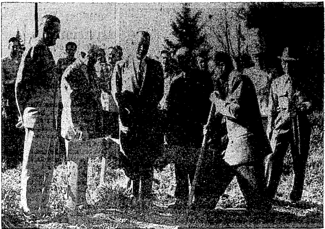
Idaho's new music building is under way. Hall Macklin, head of the music department, has the honor of turning the first shovel of earth. Looking on are (left to right) President J. E. Buchanan, T. S. Kerr, dean of the college of letters and sciences; Hugh Richardson, Lewiston architect; Carl Claus, director of the university orchestra, and George Gagon, university engineer. In the background are music students taking time out from classes for the event.
