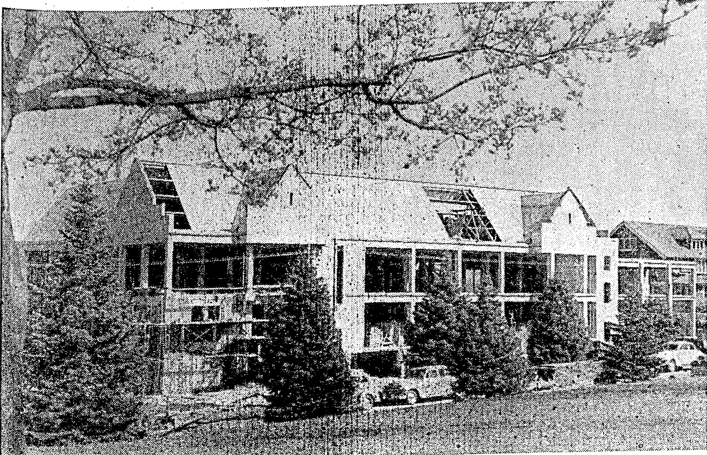
NEW MUSIC HALL —Not yet completed, but well on the way is the new three-story Music building. This is the last of the "Big Five" construction program for which the 1949 state legislature appropriated funds. The building will be ready for use next fall.
