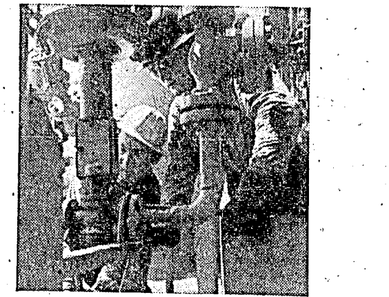
MAINTENANCE TEAM making a speedy change of a methanol valve to minimize production loss.
