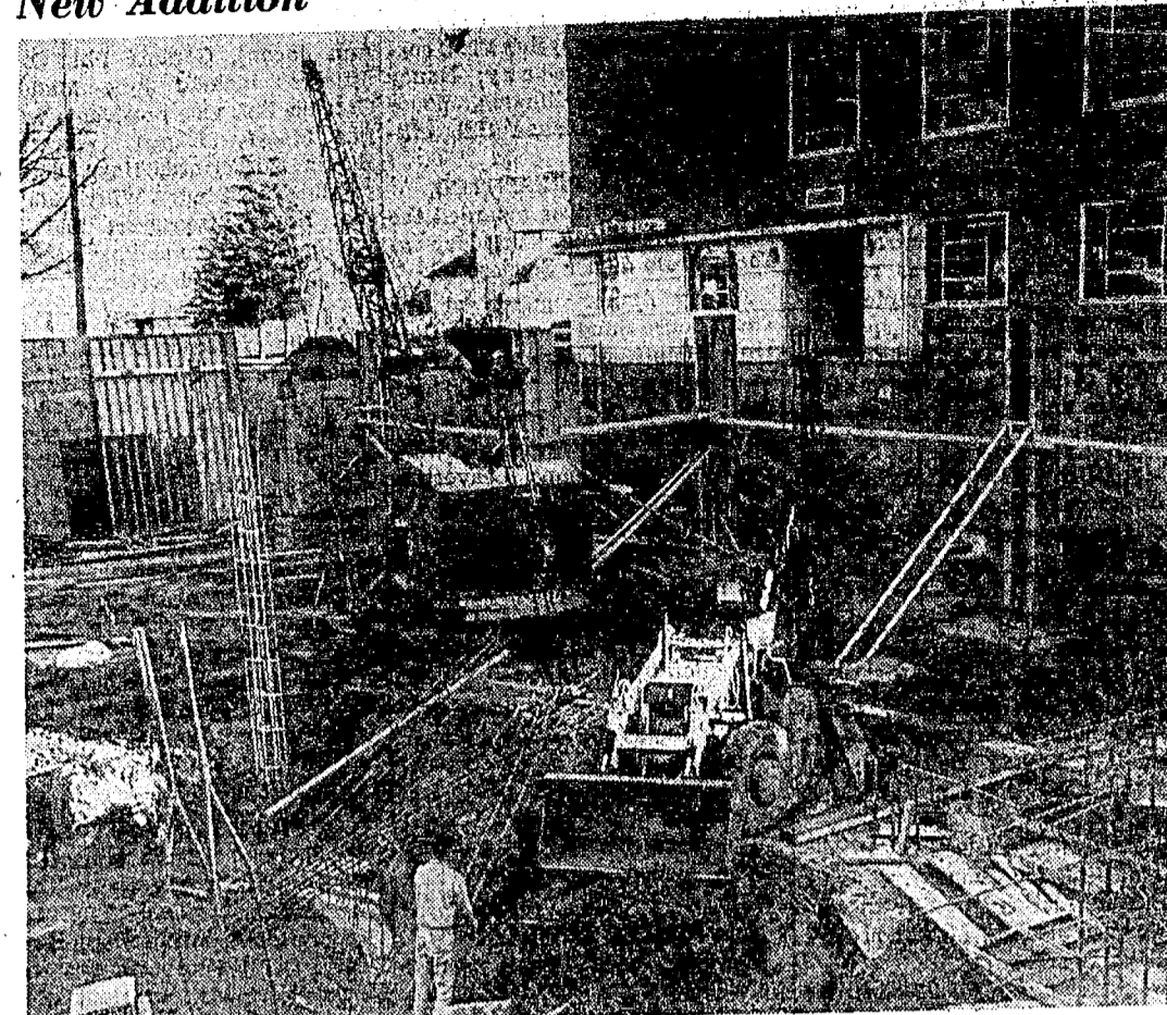
CONSTRUCTION of the new Student Union Building addition was started last October. When finished, ASUI activities will move in the new wing while the old portion of the SUB is being revamped. The SUB will be twice its present size when the building is completed.
