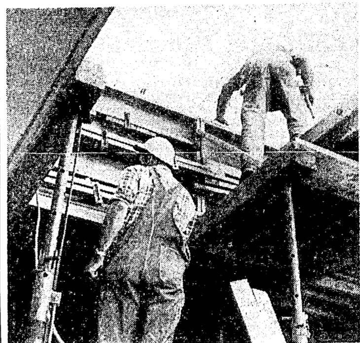
SUB CONSTRUCTION PROGRESSES . . . Two workmen are shown working on the roof of the first floor which was poured yesterday. Construction is proceeding slightly ahead of schedule which calls for opening of the new addition next fall. (Bruce Dunn photo.)
