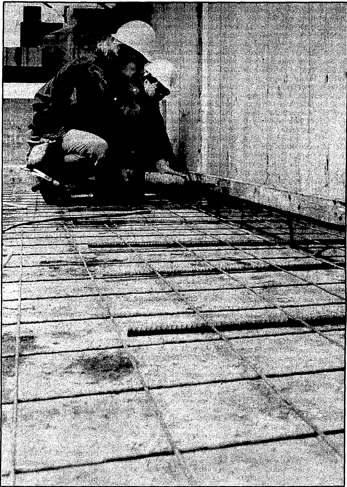
Mark Lloyd on the left and Mike Allen of Ponco Construction prepare to pour a slab of concrete on the new addition to the Physical Science building Monday. (Jim Vollbrecht PHOTO)
