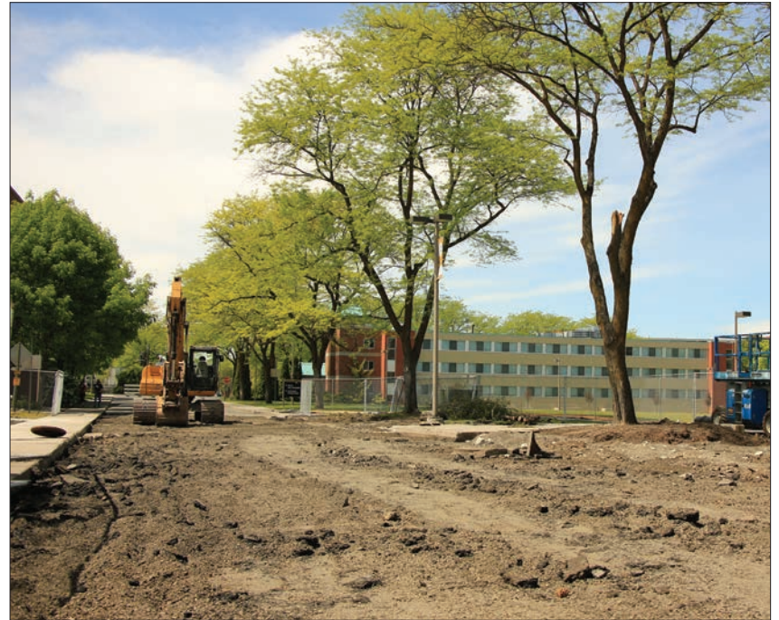
Construction workers clear out a section of 6th Street for a new traffic calming project similar to last year's addition to Deakin Street.
