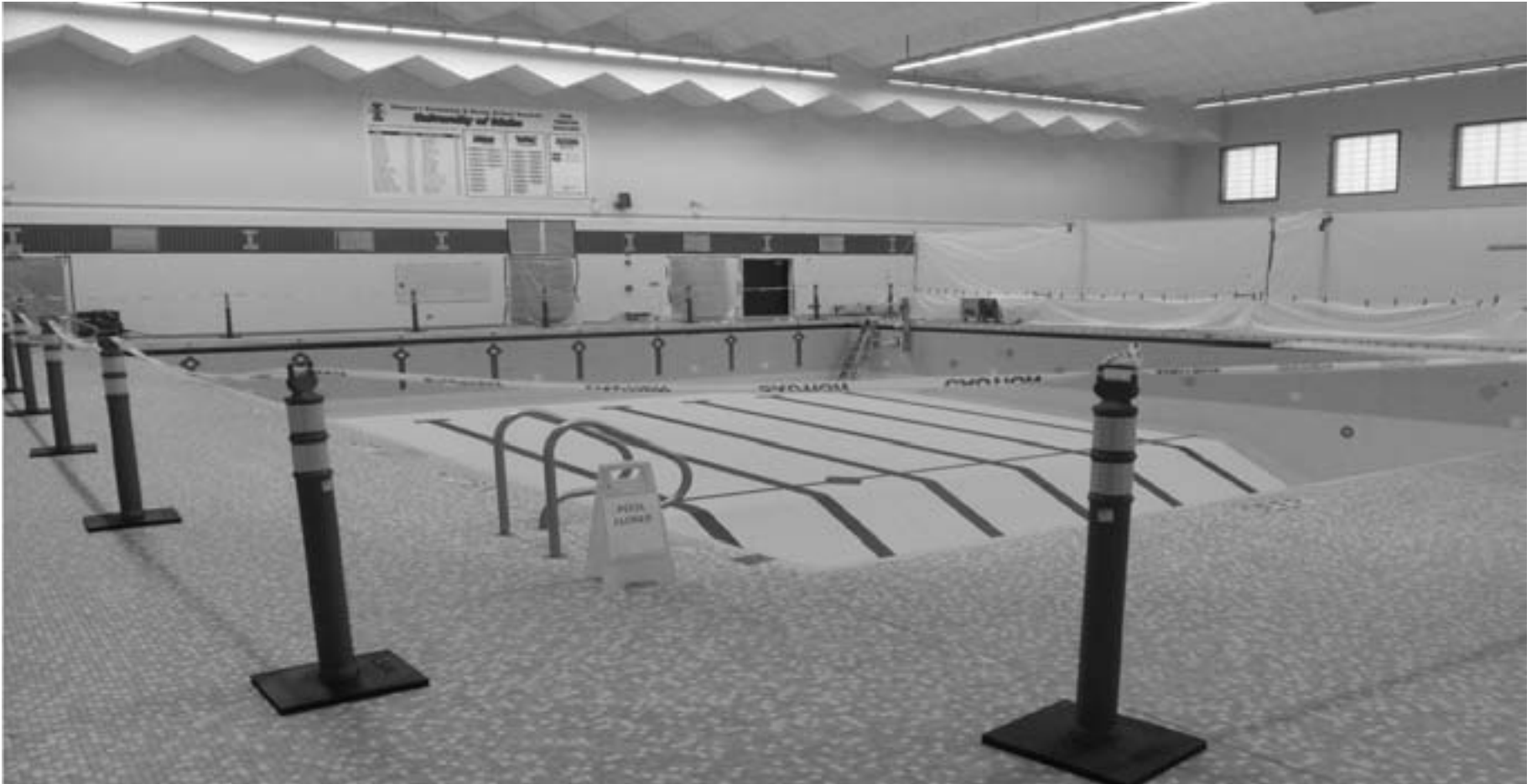
The University of Idaho Swim Center undergoes renovation during the summer. The renovations began May 8 and will conclude Sept. 8.
