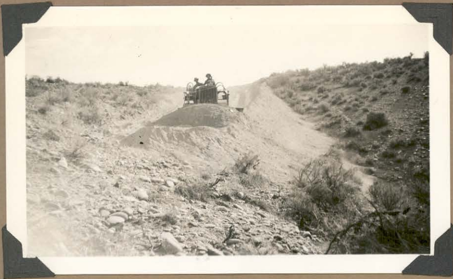
A sample of heavy road construction by DG#3, which reaches the heart of thousands of Acres of range-- A boom to the stock industry of Owyhee County.
