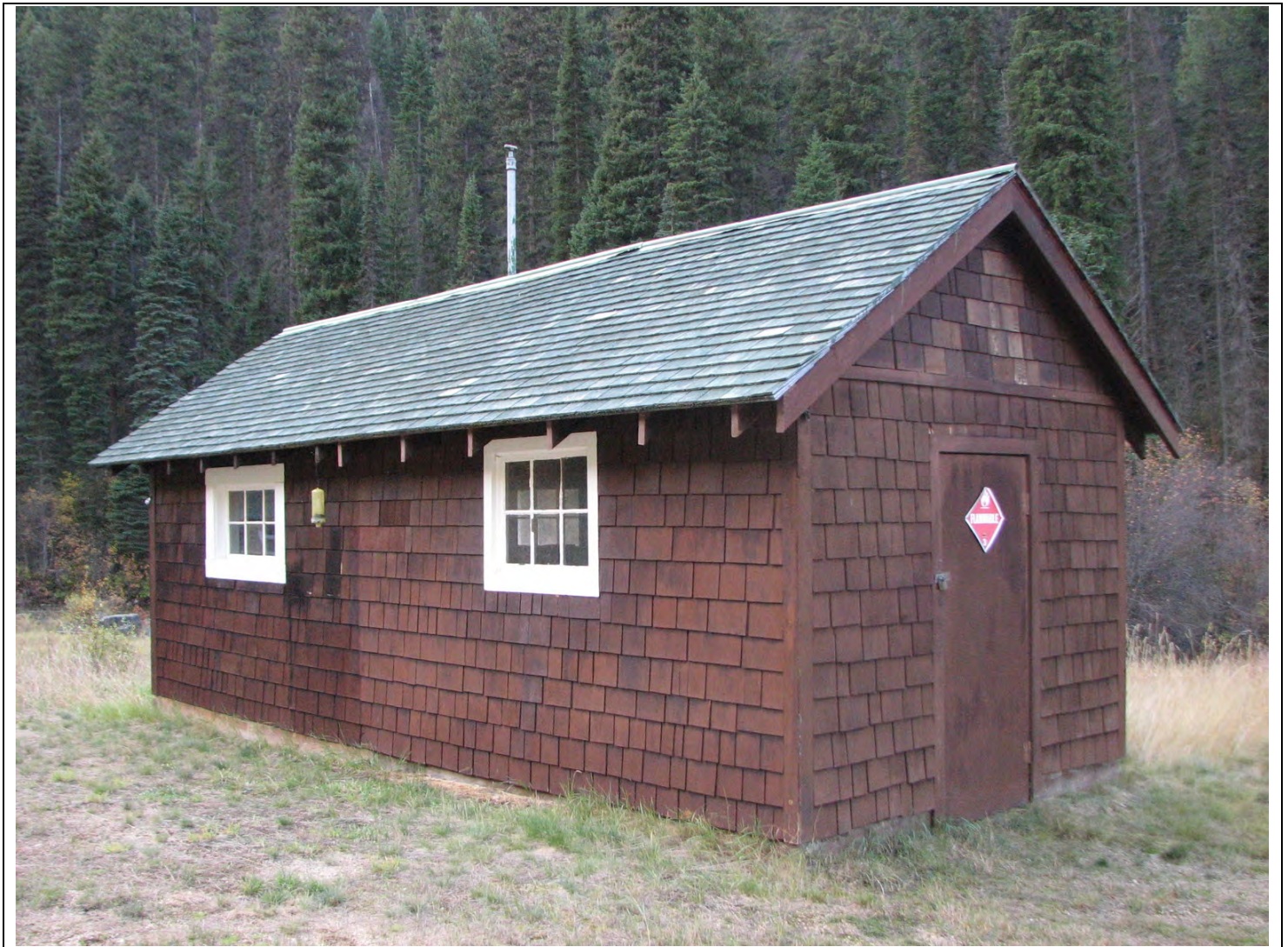
Photo 0020 Looking southwest to the east (side) and north (front) walls of the flammable materials shed.
