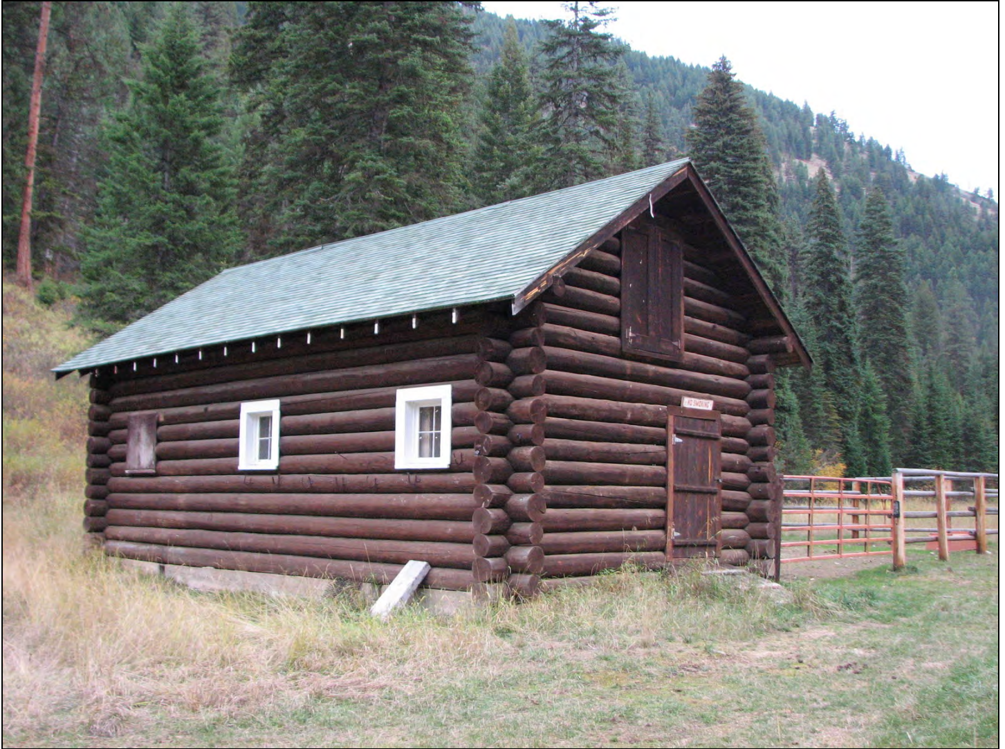
Photo 0022 Looking southeast to the north (side) and west (front) walls of the barn.
