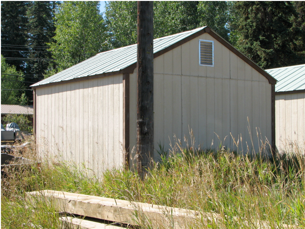
Figures 19a and 19b. The south and east sides (top) and the east and north sides (bottom) of Building 5, the East Storage Building (#1401), McCall District Administrative Site, 2008.
