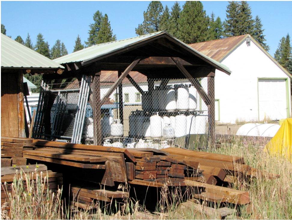
Figures 14a and 14b. The north and west sides (top) and the south and east sides (bottom) of Building L, the Propane Storage Building (#1377), McCall District Administrative Site, 2008.
