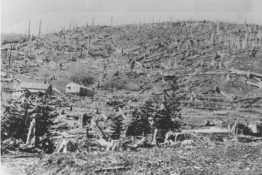
Figure 20. Camp Lookout Mountain under construction 1933. Note wood frame structures at top of camp on stilts. Mess hall under construction. Courtesy of Gifford Pinchot National Forest Heritage Program.
