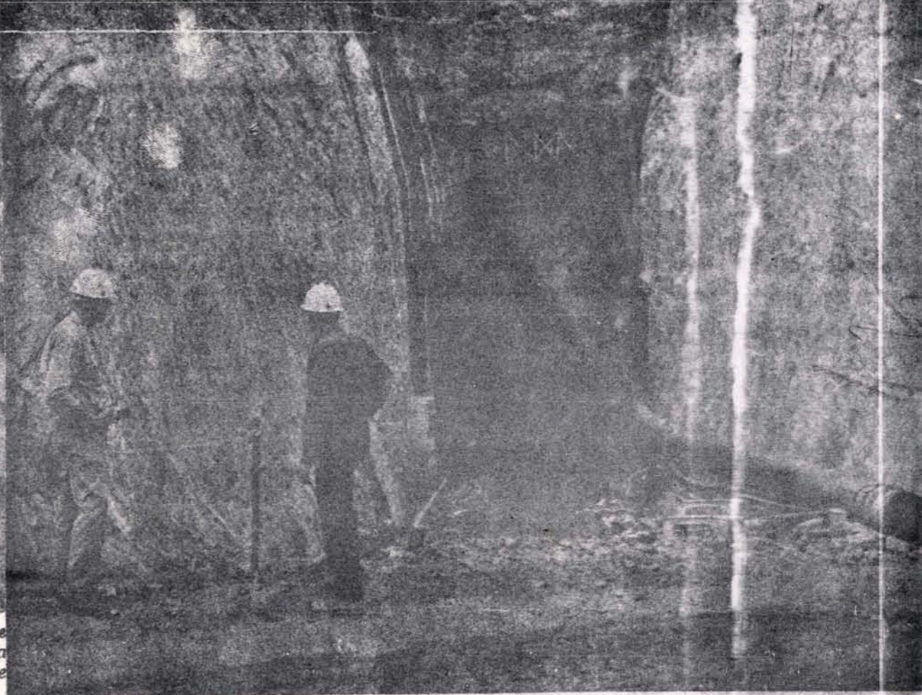
Orofino Mayor A. B. Curtis, left, and Robert D. Owsley, project engineer for the Army Corps of Engineers, inspect the beginnings of the 1,700-foot diversion tunnel that will carry the North Fork of
