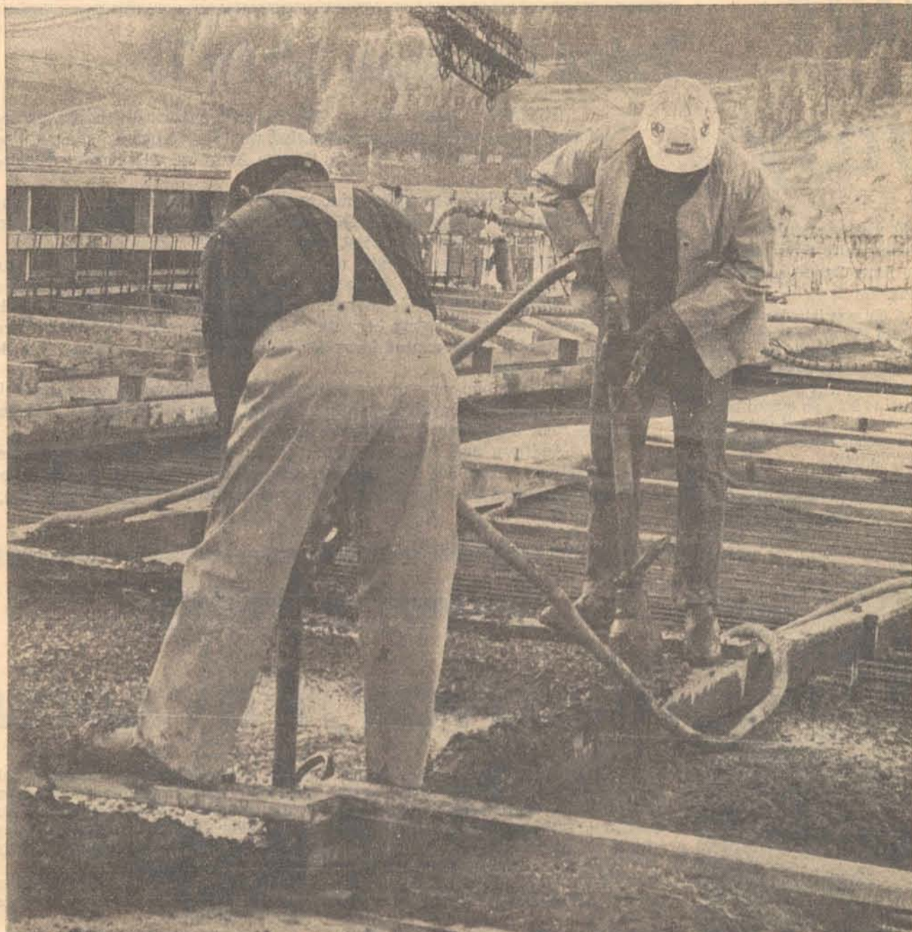
Jerry Gore, left, and Luis Uriarge, employes of Dworshak Dam Constructors, vibrate concrete down through steel reinforcing rods — the last time they will have to do that job. The final bucket of 6.6 million cubic yards of concrete was poured yesterday for the main structure of the 717-foot high dam near Orofino. The two are working on a portion of the roadway deck atop the dam.
