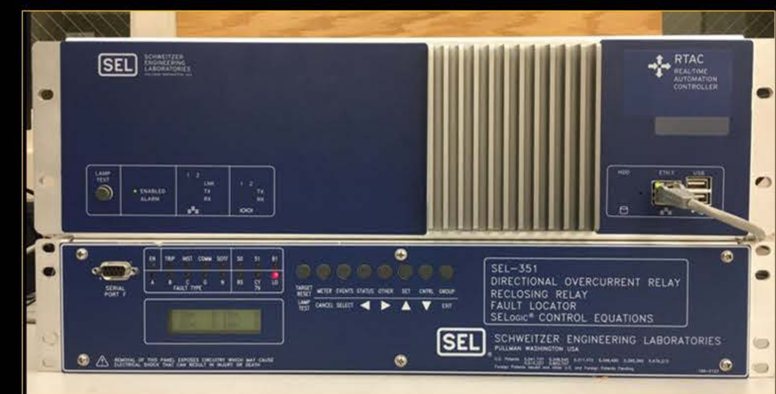
SEL RTAC atop SEL-351 Team members used the SEL RTAC as an RTU. The device can manage equipment remotely. In Lab 4, the RTAC controls and receives data from the SEL-351 protective relay.
