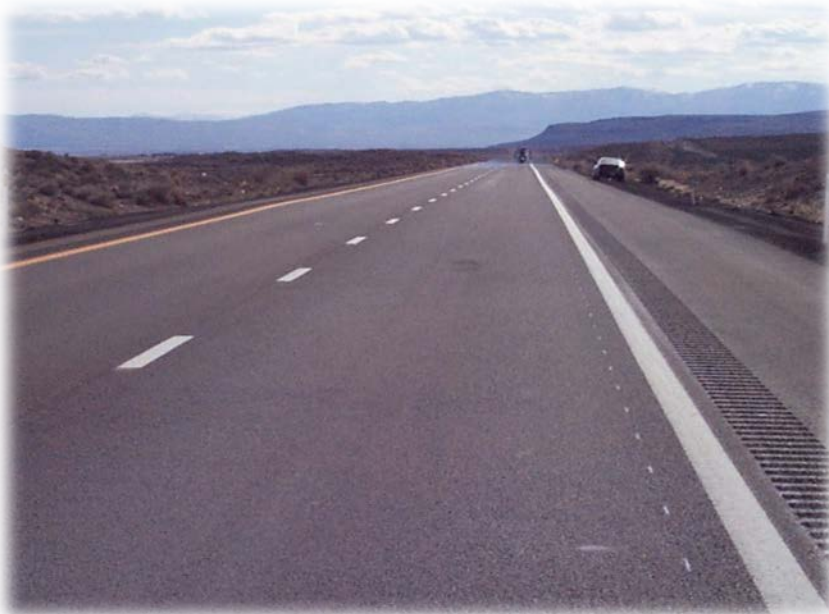
PG 64-22 modified, no rutting
