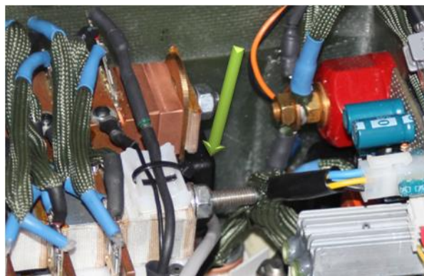
Figure 78: Current Sensor Location in the Battery Box
