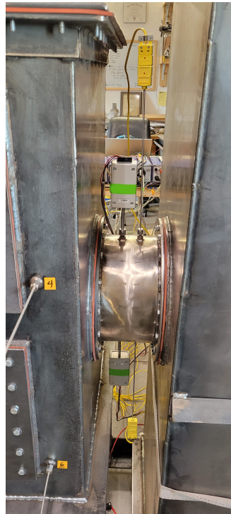
FIGURE 4.18: Placement of thermocouples and velocity sensors on the upper and lower section of the axial cross-vessel duct.
