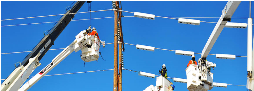
Figure 2.11: Inductive D-FACTS Devices Installed on Transmission Line [12]
