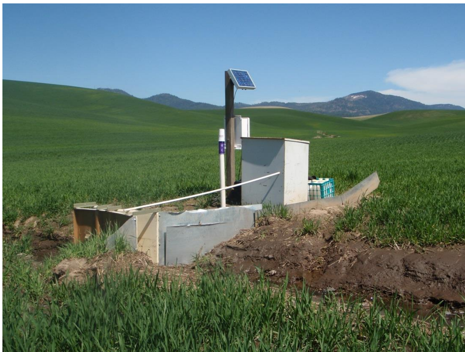
Figure A.1 Photo of the instrumentation at the Idaho-CT site.
