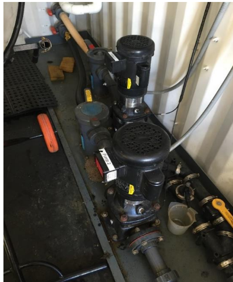
Figure 7: Influent Pumps #1 and #2
