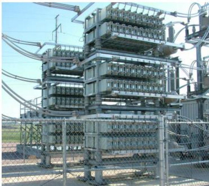
Figure 1-1 Shunt Capacitor Bank [1]
