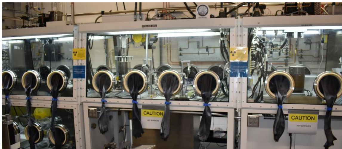
Figure 3.5. Fuel Cycle Glovebox in FCF with bench-top furnace (right end of box).
