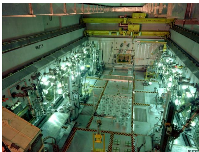
Figure 3.1. Bird's eye view of the main cell in HFEF.
