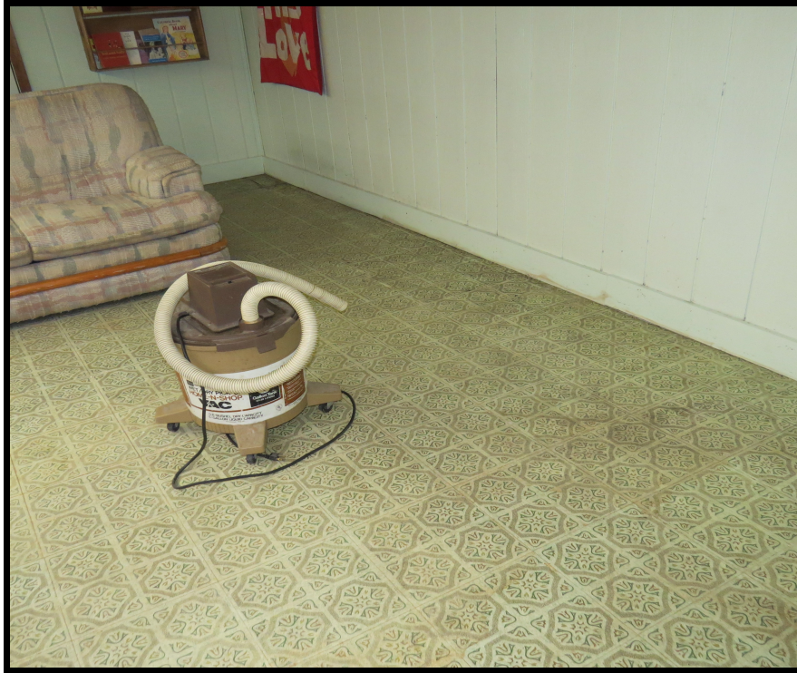
Figure 61: Water damage and a shop vac left from a previous flooding (Kleer-Larson 2016)
