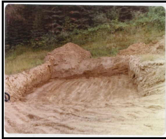
Figure 30: The hole that would become the basement of Our Lady of the Woodland (Triplett 1980)
