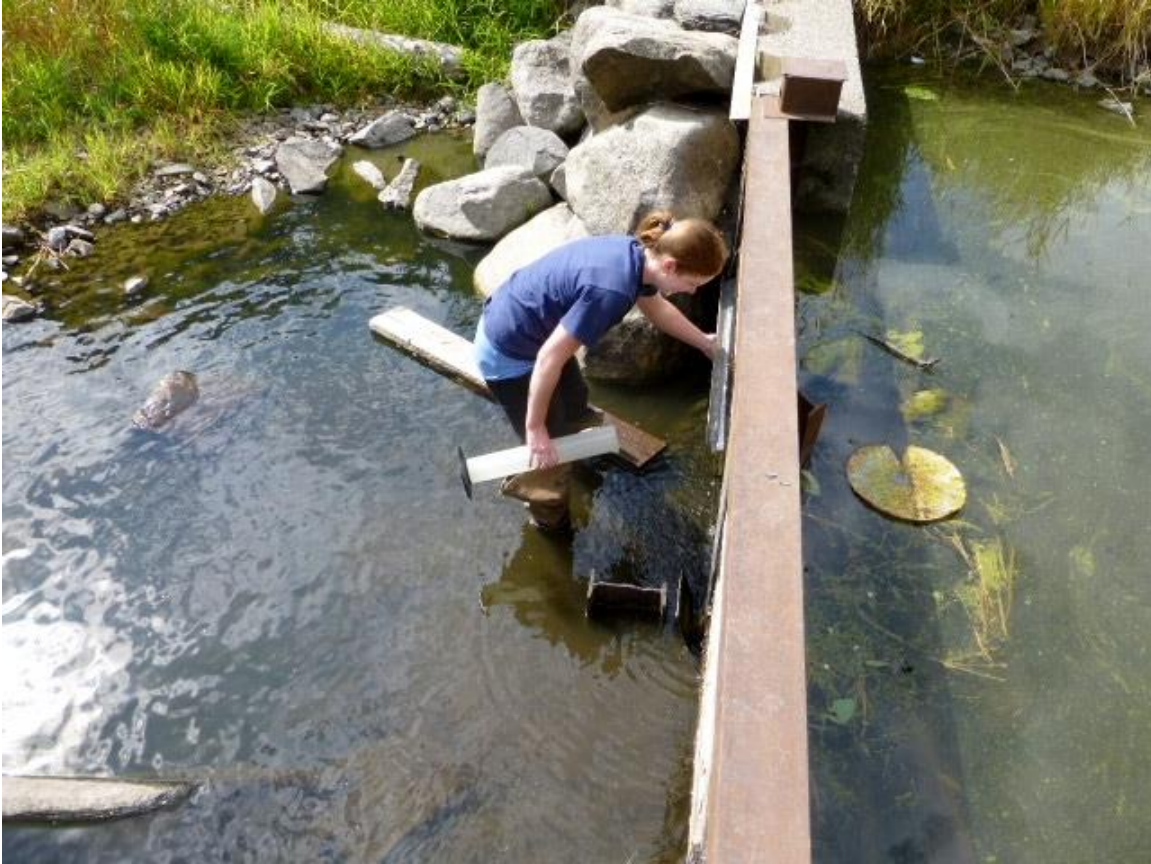
Figure B.7: Image looking down on the dam when it is in place. Leakage was measured with a metal piece, 2L graduated cylinder and a stopwatch. Two measurements were taken, one from the left side and one from the right. The metal piece is placed against the side of the dam and funnels water into the cylinder.
