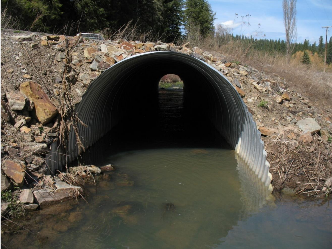
Figure B.2: Culvert on the opposite side of the road from the North side box location. This is where cross section and velocity measurements were taken starting from the left side of the culvert. The culvert was marked on the underside beginning at 0.1 meters to 1.85 meters from left to right.
