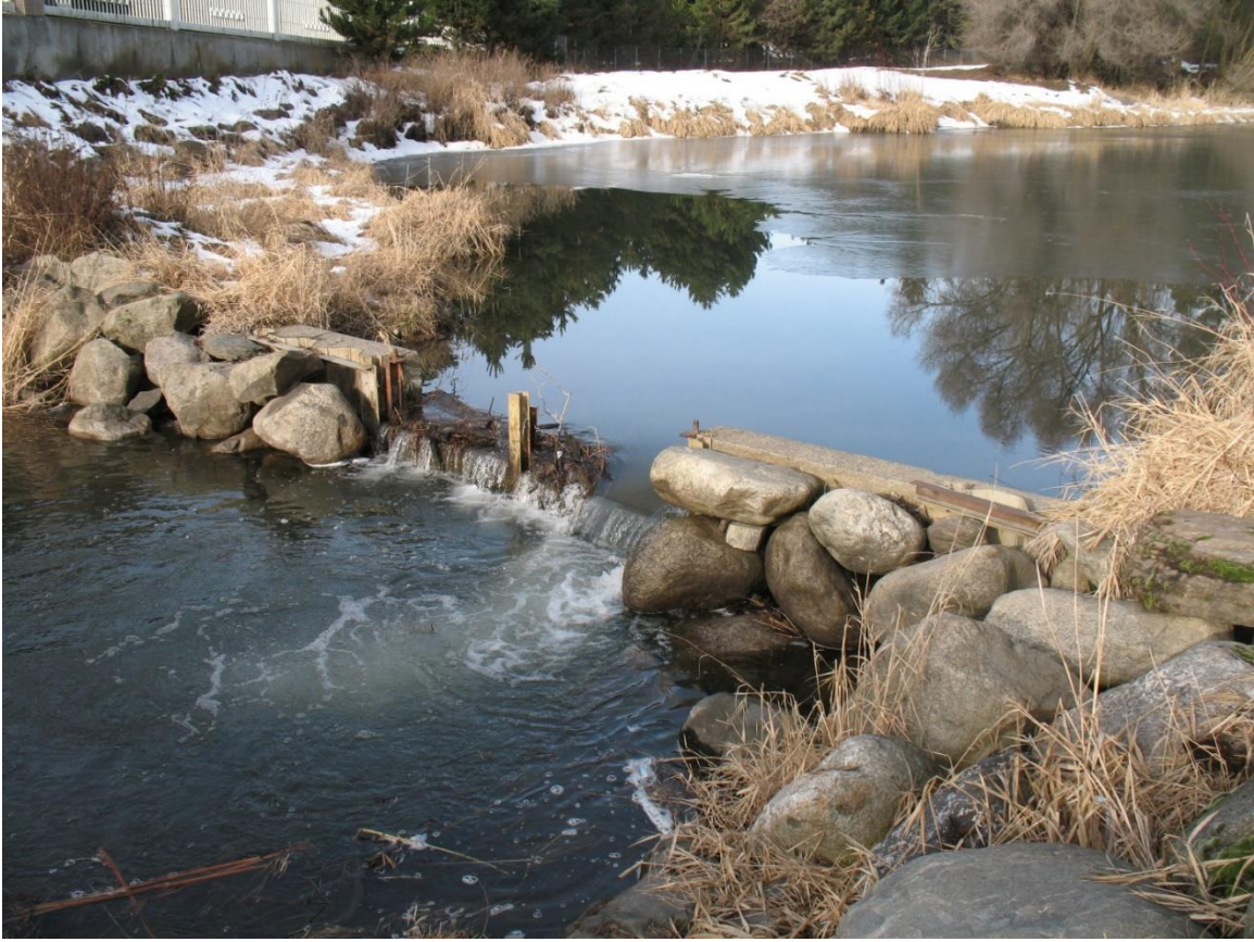
Figure B.6: Image of the Outflow location with the dam removed. Discharge was measured by spreading a tape across the opening of the dam and measuring velocity from the left side (looking downstream).
