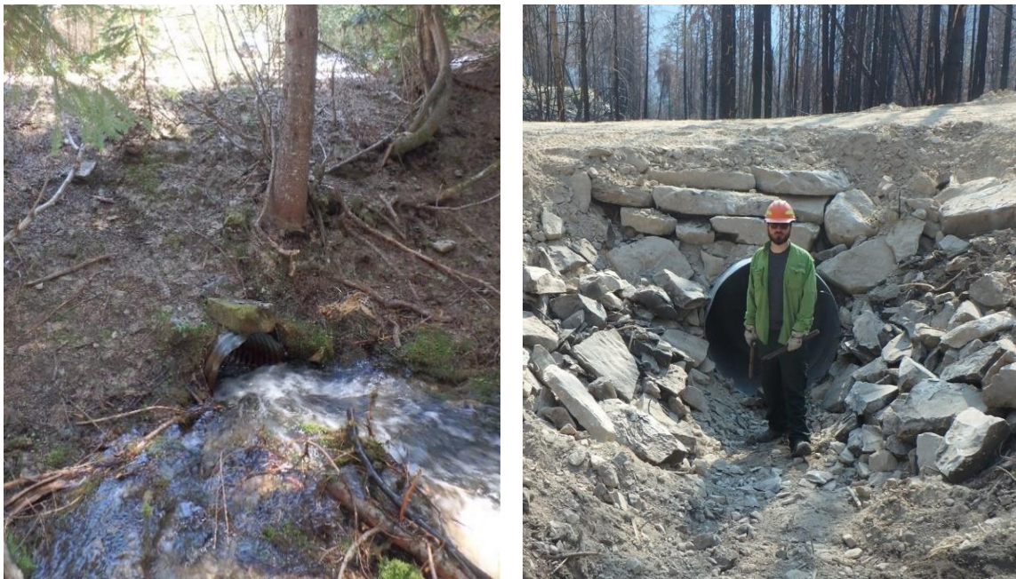
Figure 2: Example of undersized culvert (left) and post-fire upgraded culvert (right).
