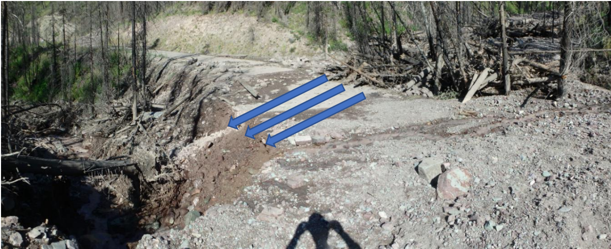
Figure 1: Debris flow at Spruce Creek following the 2017 Rice Ridge fire on the Lolo National Forest in Montana. Notice the large amount of woody debris on the upstream side of the road which blocked the culvert and redirected the flow onto the road surface.
