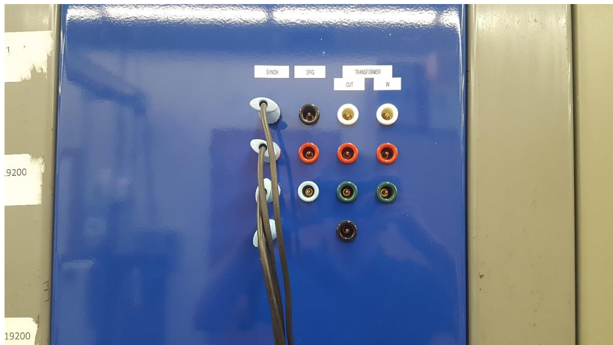
Figure 27: Connection Panel On AMPS System Above Computer
