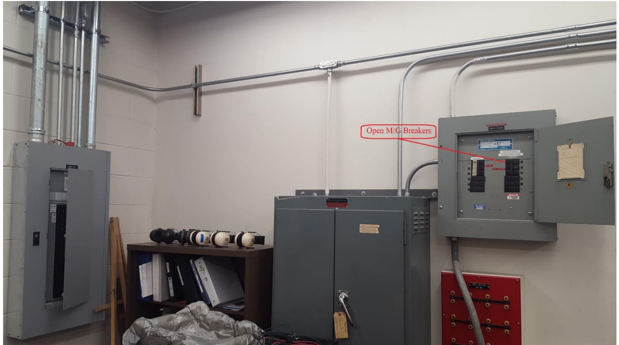
Figure 29: Breaker Box for AMPS MG set
