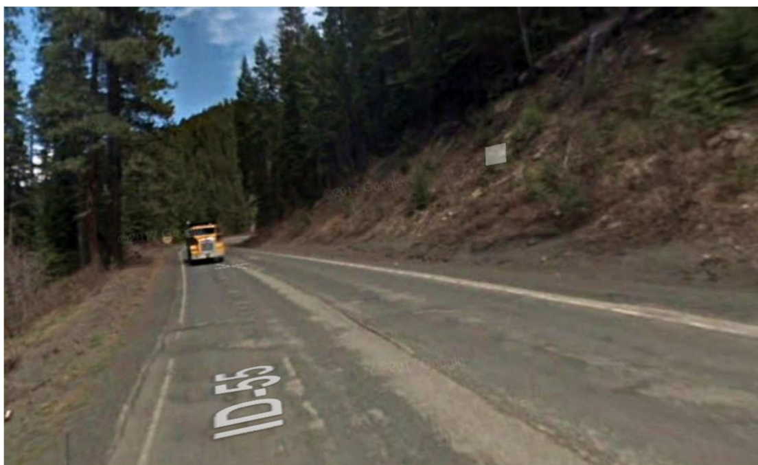
Figure 1.1. Road with a poor pavement marking condition
