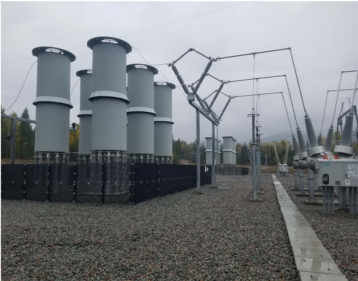
Figure 3.2: Reactor banks at Noxon substation with one bank in the foreground and the second bank in the background
