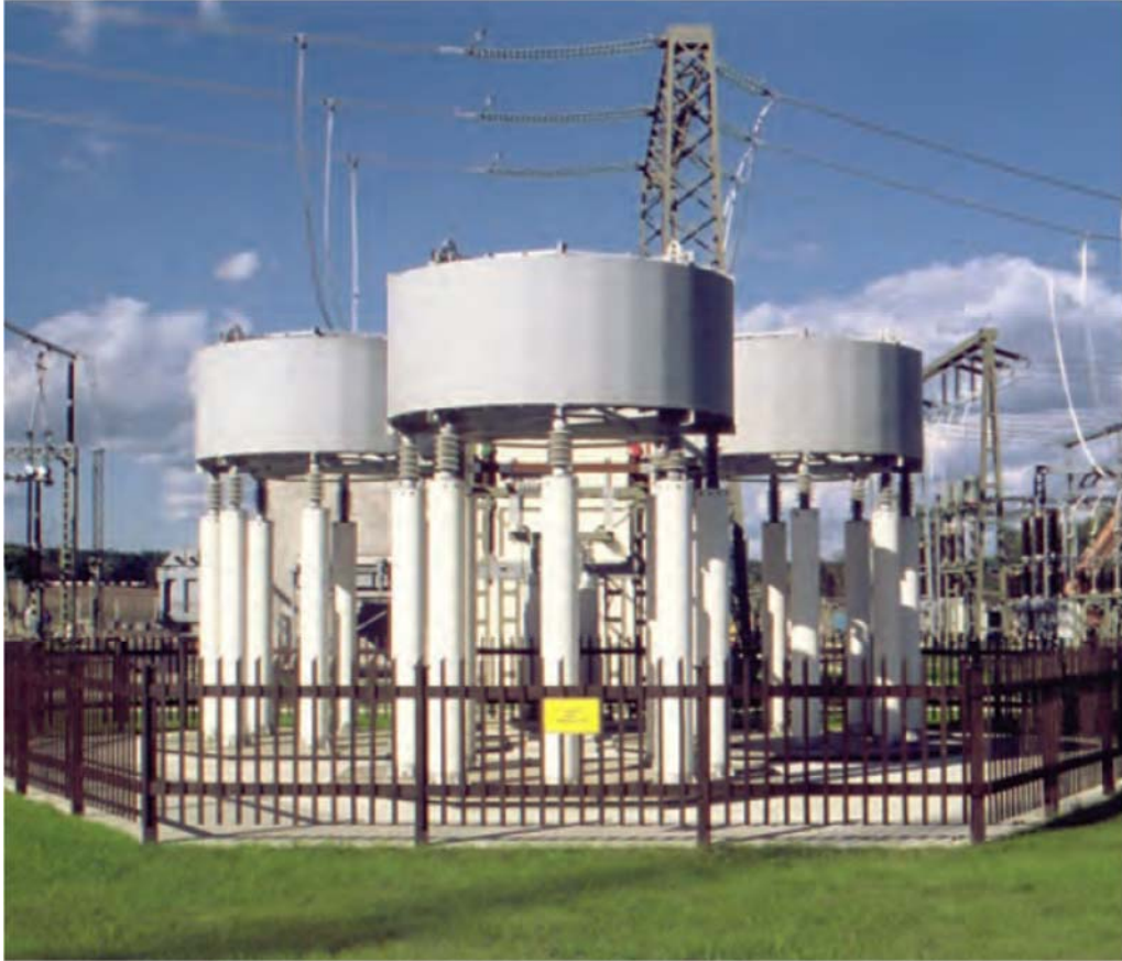
Figure 2.1: 20kV, 45MVAR air core reactors mounted on insulators and pedestals [4].
