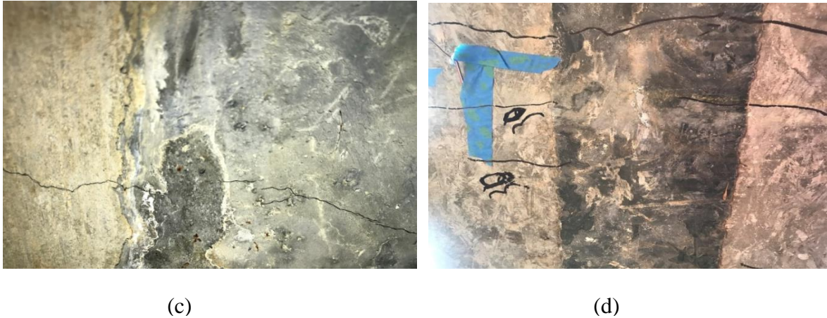
Figure 2.20. (a) Crack pattern observed in flexure, BC-1 (b) Crack pattern observed in flexure, BC-2 (c) Cracks at the bottom surface of the hybrid connection, BC-1 (d) Cracks at the bottom surface of the hybrid connection, BC-2
