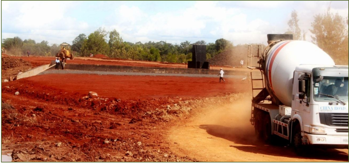
Photo 9: A section of the Nairobi Southern Bypass under construction in Karen area
