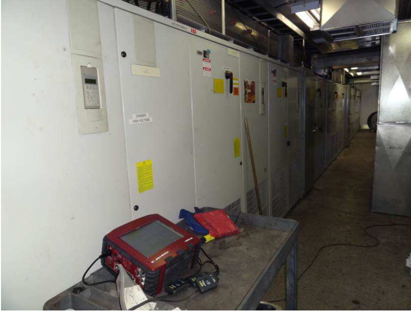
Figure 34: ABB CCS DTC Drive
