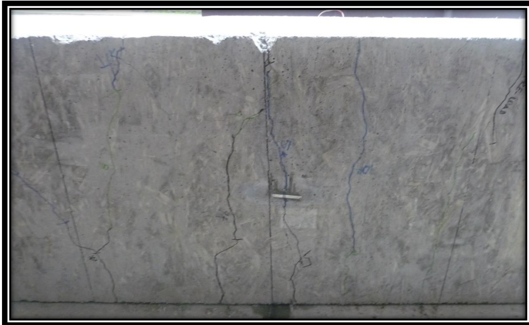
Figure 48: Segmental Connector Specimen 2—Crack Pattern (Bottom of Specimen)
