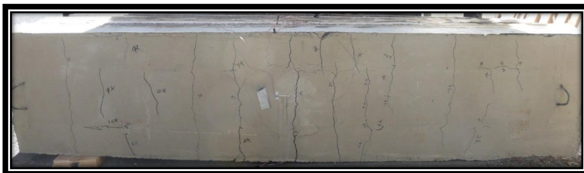
Figure 96: 10" FPCS Specimen 1—Crack Pattern (Bottom of Specimen)
