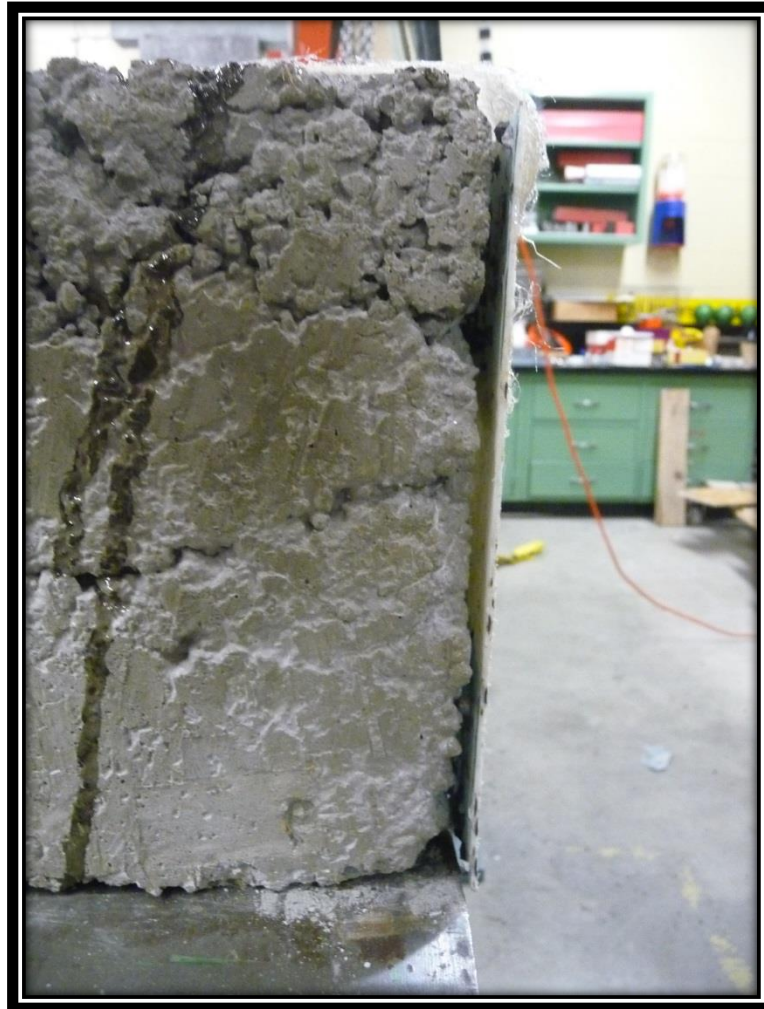
Figure 89: Debonding and Poor Concrete Vibration
