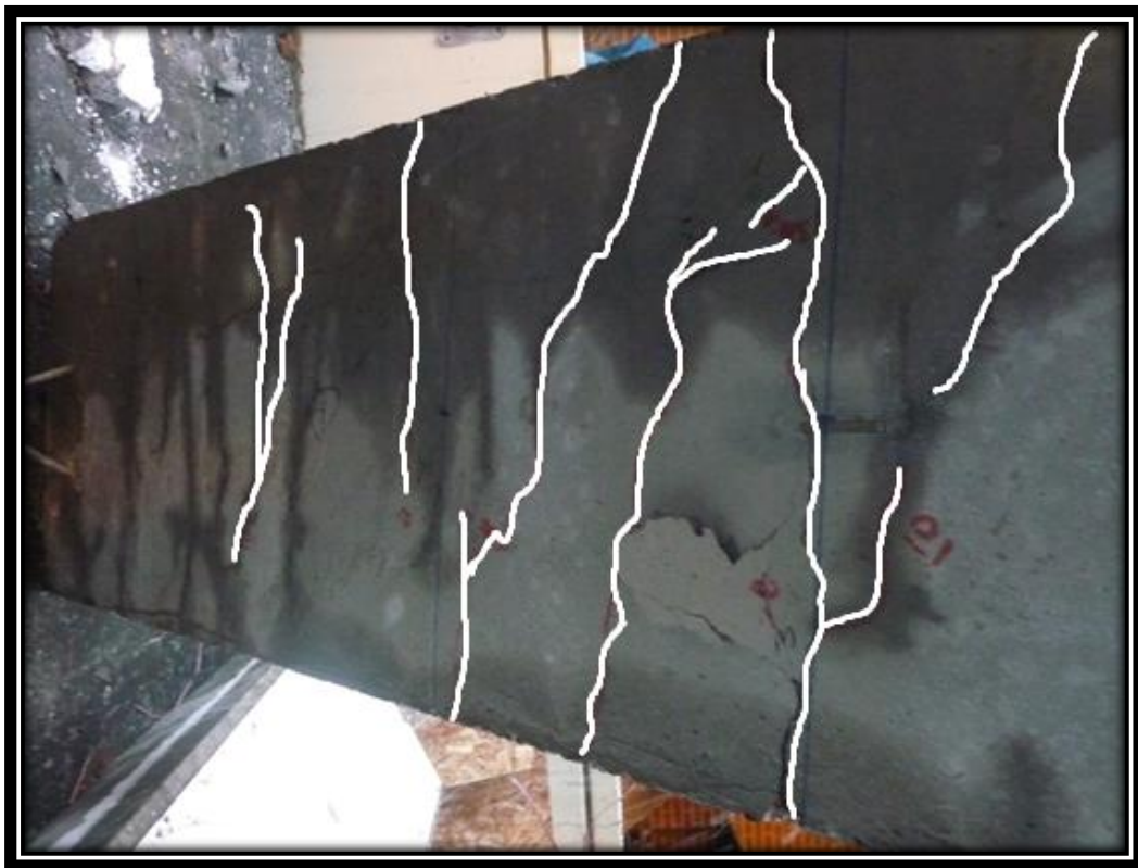
Figure 71: Segmental FPCS Specimen 2—Crack Pattern (Bottom of Specimen)
