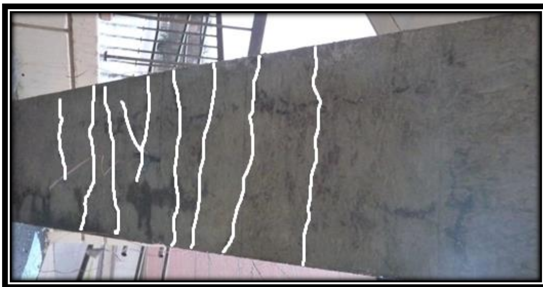
Figure 49: Continuous Connector Specimen 1—Crack Pattern (Bottom of Specimen)
