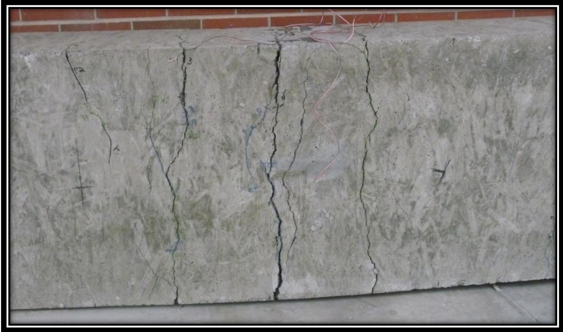
Figure 52: Solid Specimen 2—Crack Pattern (Bottom of Specimen)
