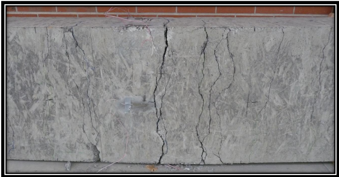
Figure 51: Solid Specimen 1—Crack Pattern (Bottom of Specimen)
