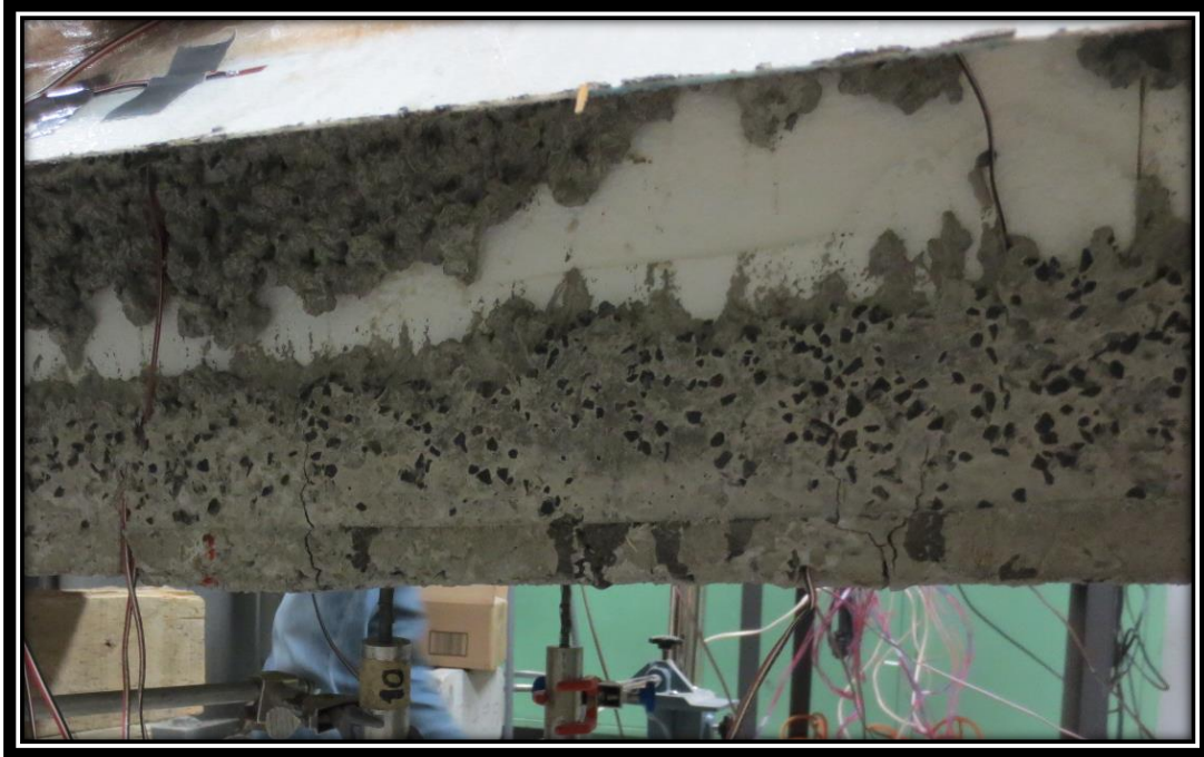
Figure 122: Full Scale 8" FPCS Cracking
