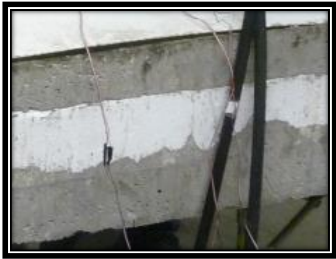
Figure 60: Debonding of FRP Top Plate
