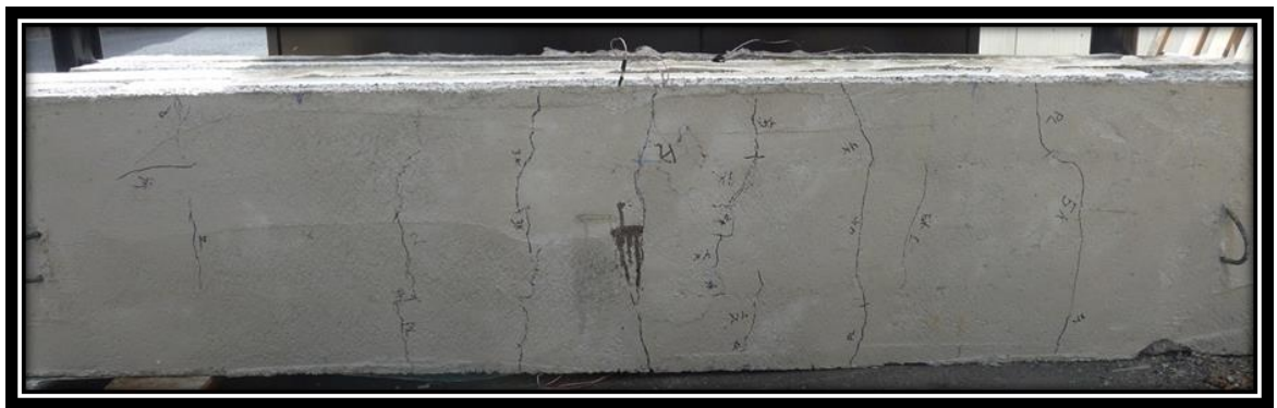
Figure 100: 8" FPCS Specimen 2—Crack Pattern (Bottom of Specimen)
