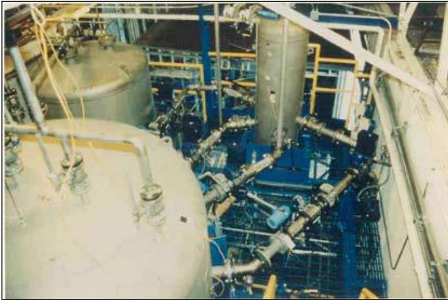
Figure 2-5: Top-down view of the PUMA Test Facility
