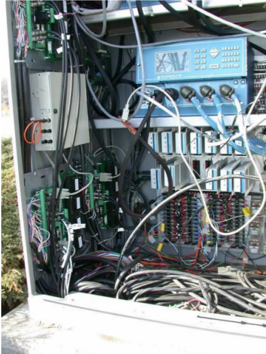
Figure 2.5: The inside of a typical traffic cabinet [29].
