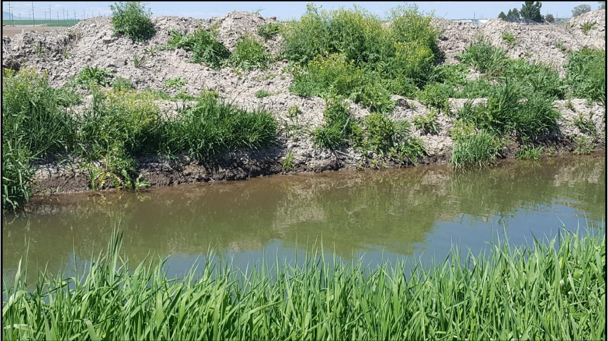
Figure 3.6: Vertical absorption of surface water by banks during high temperatures.
