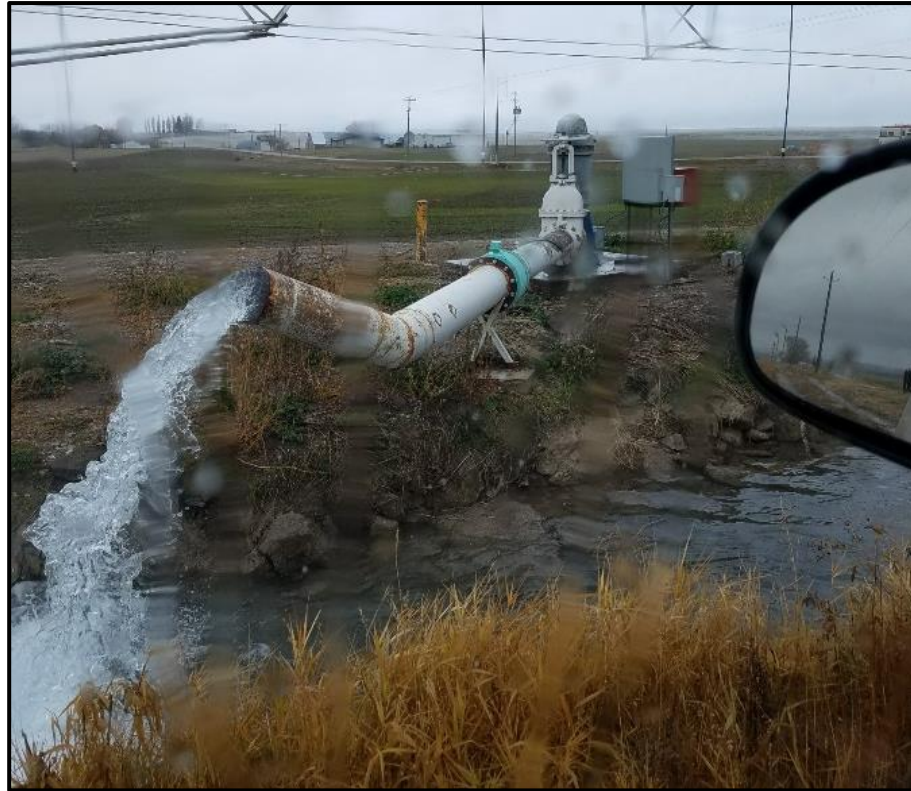
Figure 4.9: The Simm's Well during the pumping test.
