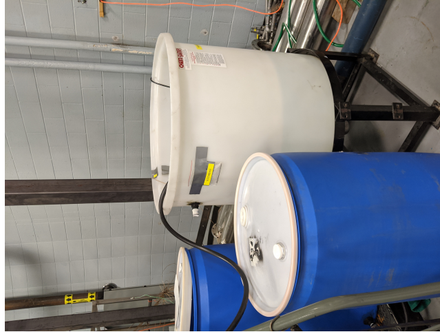
Figure 3.10: Cooling water reservoirs.
