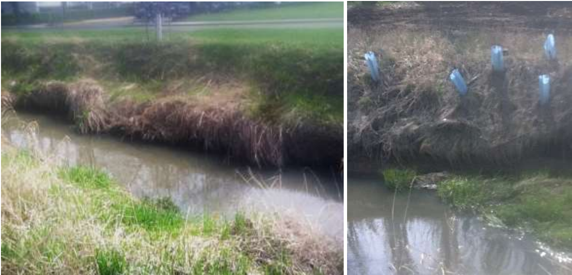
FIGURE 4.13 Example of widening processes and bank failure in recently restored section of Paradise Creek in the urban area.
