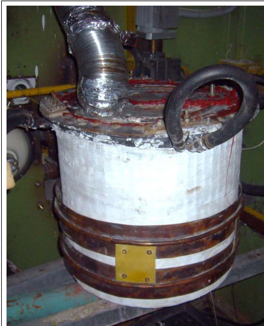
Figure 11-31. The complete assembled installation for System Optimization Test #2.
