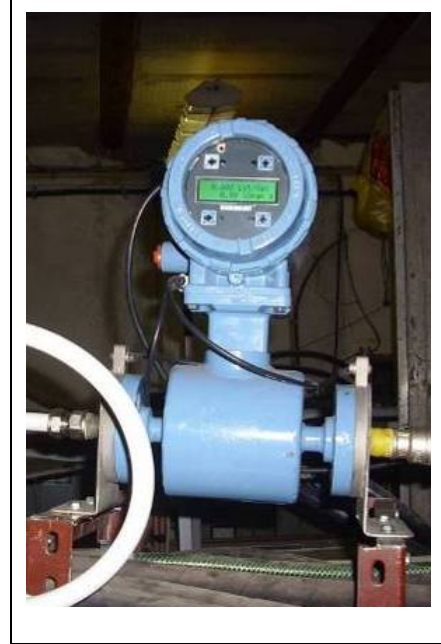
Figure 12-2. High flow, precision Rosemount flow meter.
