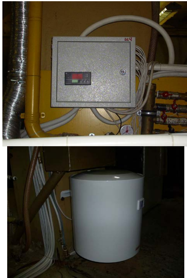
Figure C-33. Primary components of the water heating system for drain inductor cooling loop. Upper – controller, lower – heating tank.
