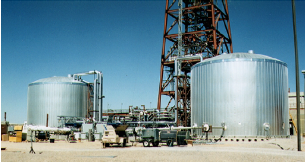
Figure 2.7: Thermal energy storage tanks at the Solar Two plant. On the left is the cold tank, and on the right is the hot tank. [26]
