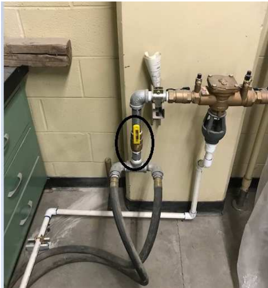
Figure A-1: Pump Coolant Water Valve Open
