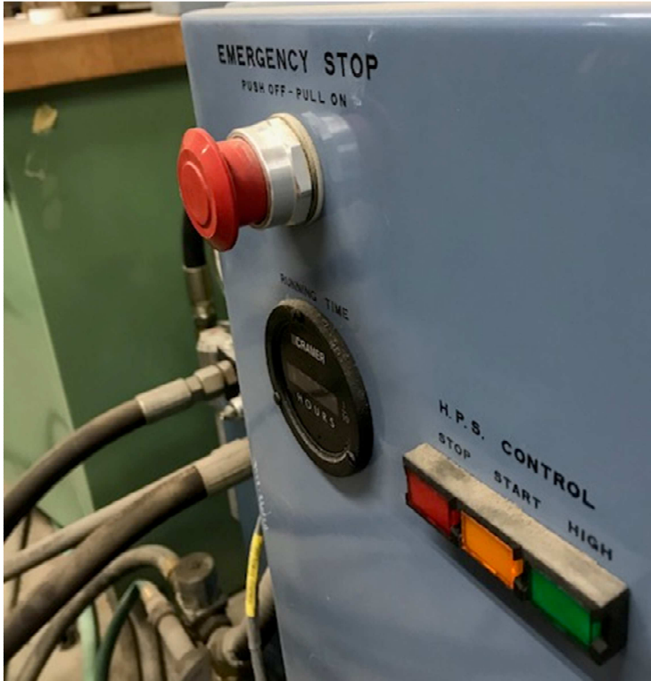
Figure A-4: Shore Western Pump Emergency Stop Button
