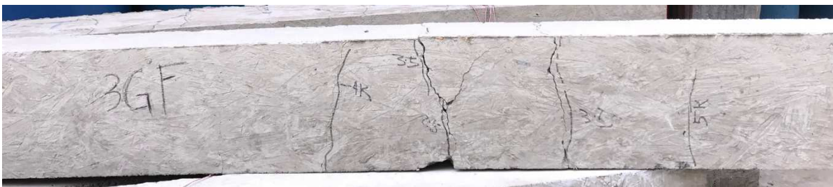
Figure 4-8: Beam 3 GF Cracked
