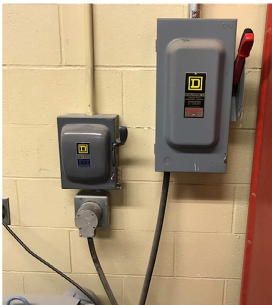
Figure A-2: Pump Power Switches On
