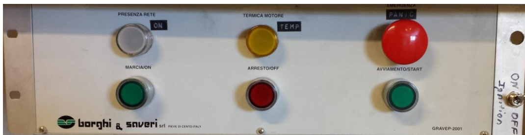
Figure 20: Starter controls inside control room.
