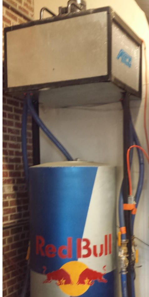
Figure 19: Red bull cooling tower and radiators.
