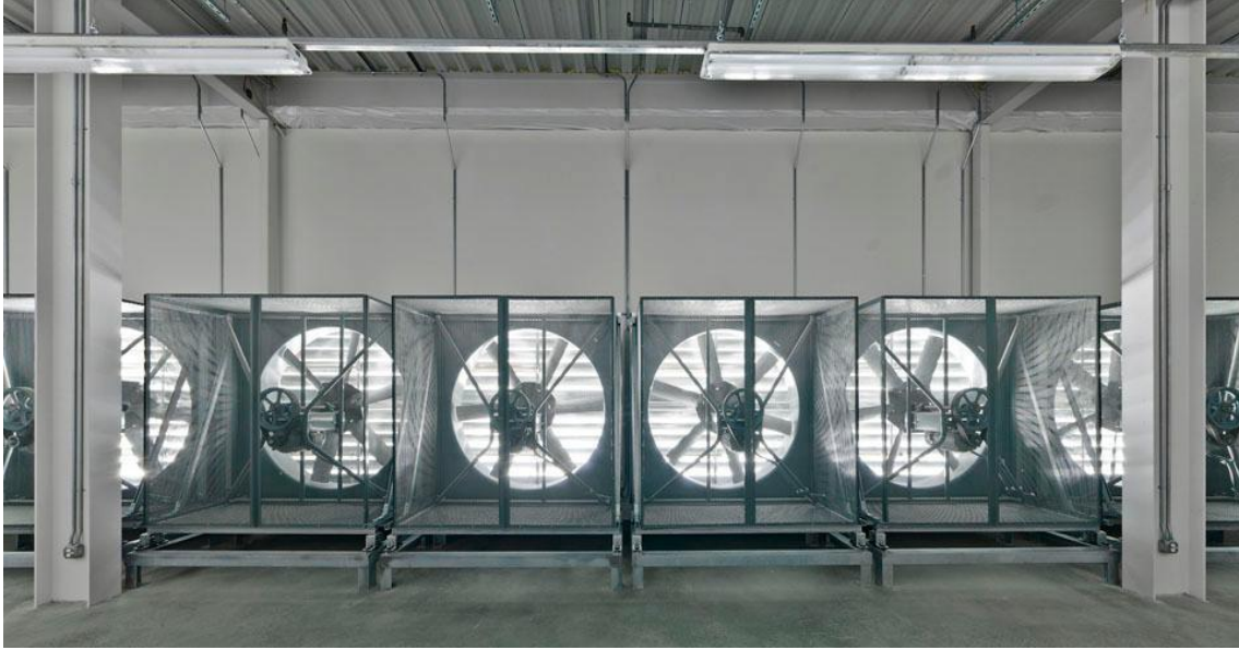
Figure 2-11: Prineville Facebook Data Center Cooling Fans [37]
