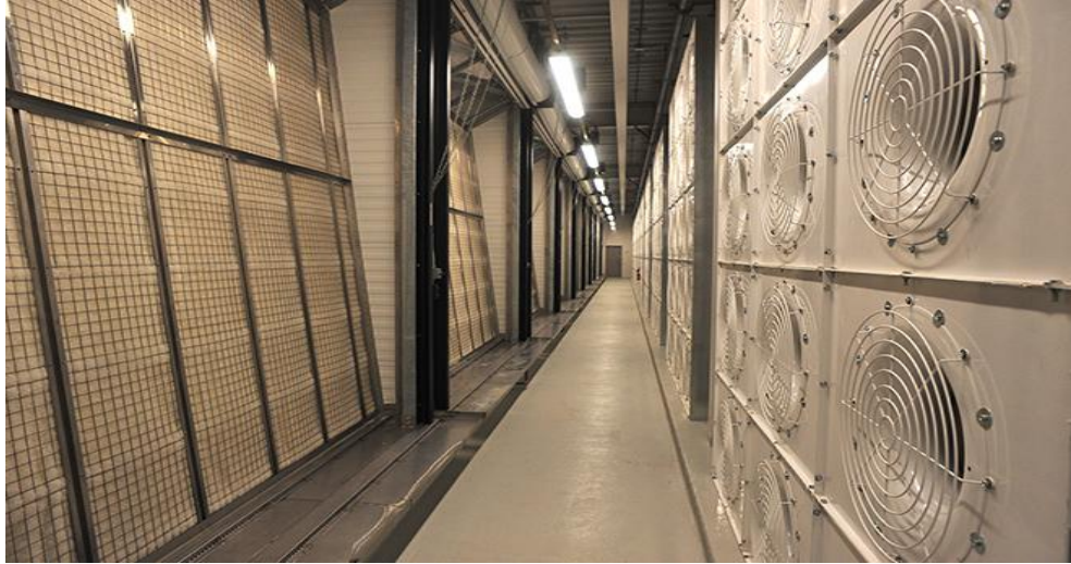
Figure 2-1: Evaporative Room in Facebook's Prineville Data Center [25]
