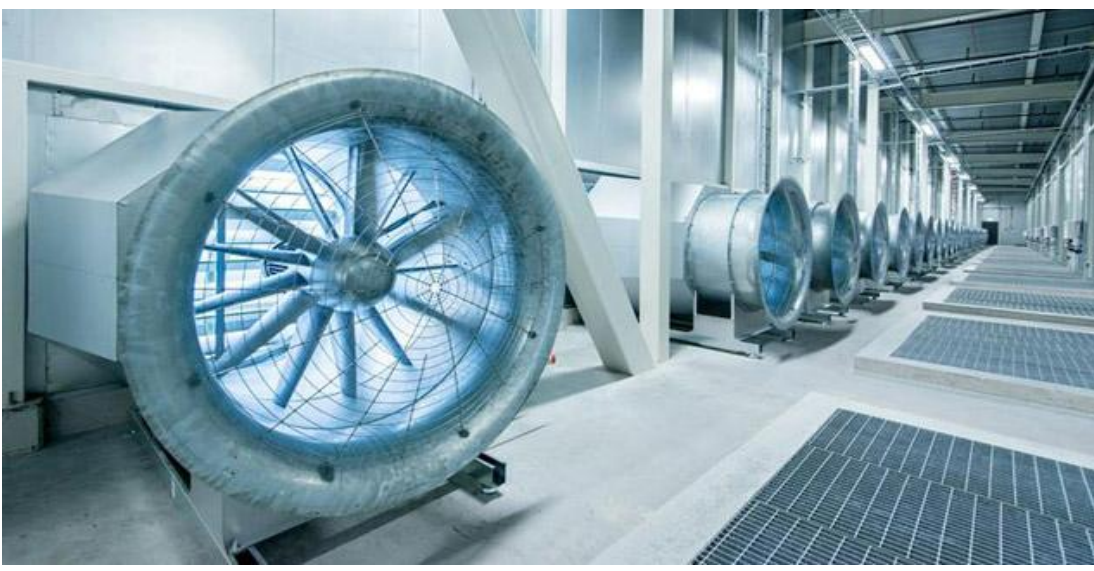
Figure 2-10: Lulea Facebook Data Center Cooling Fans [36]
